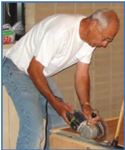
Ron Freimark calls on his carpentry skills while installing flooring on the new altar.
