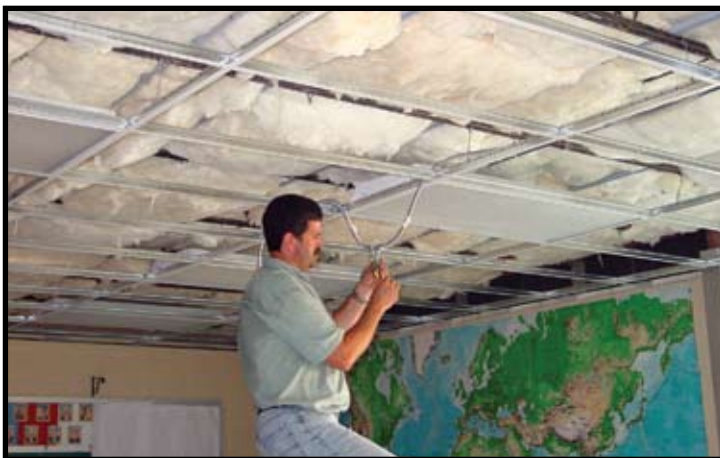
Pat Daily wires a lighting fixture in one of the newly insulated classrooms.
